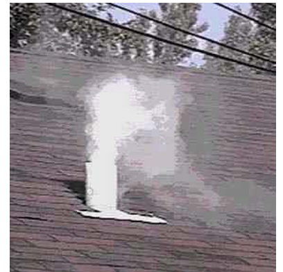
During the testing, smoke will escape from roof vents. That's normal and indicates the smoke has worked its way through the sewer system.
