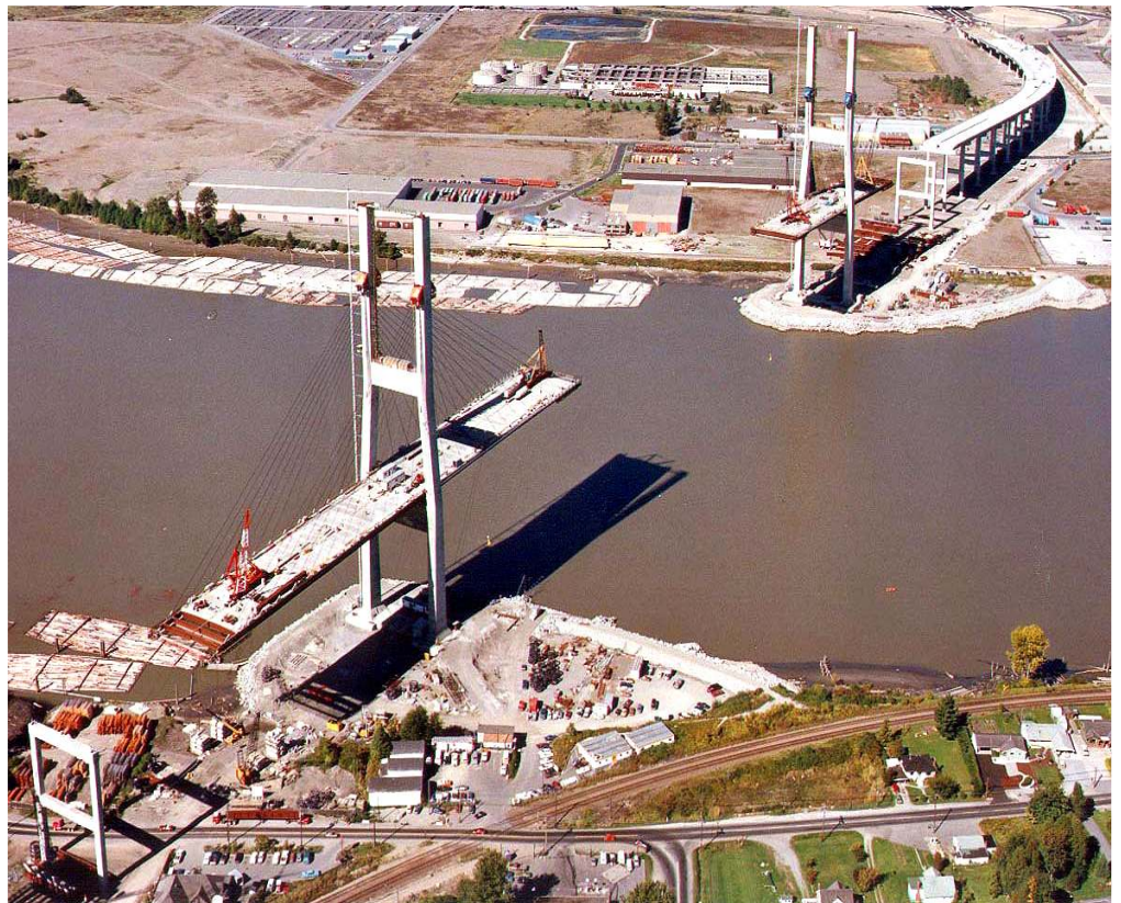
FIGURE 3: All eight "work stations" are evident at the tower-heads coupled with the four derricks at the leading edges of the balanced deck erection.
