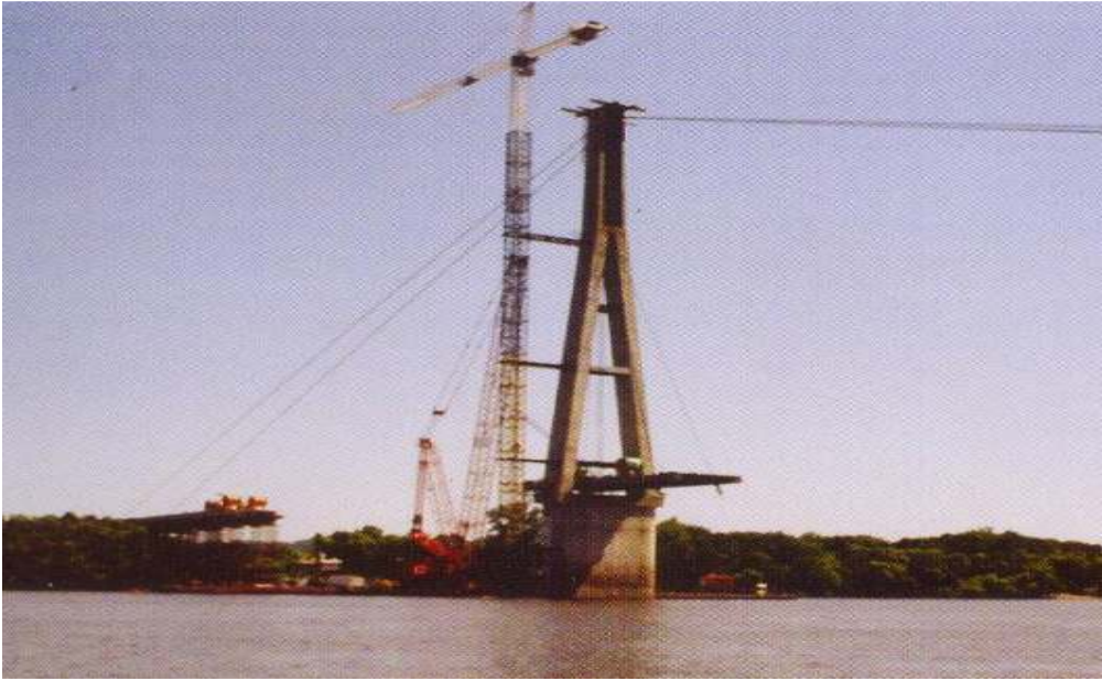
FIGURE 2: Ohio shoreline view of the guyed, 278.83' tall concrete pylon atop the 87' high, existing, main river pier.
