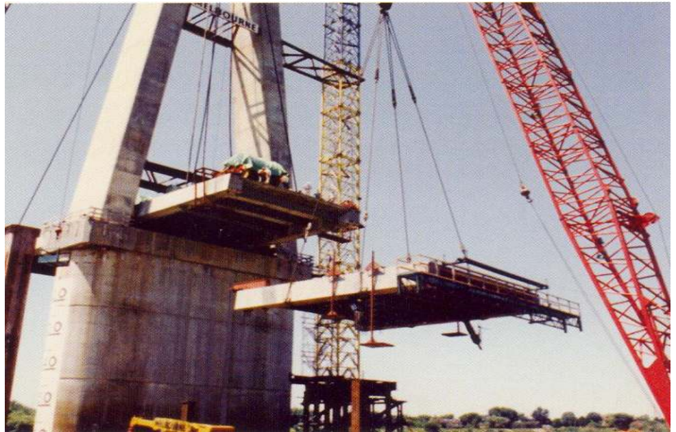
FIGURE 4: Barge mounted crane hoists 275 ton, pre-cast concrete, deck segment with alignment tongue in view
