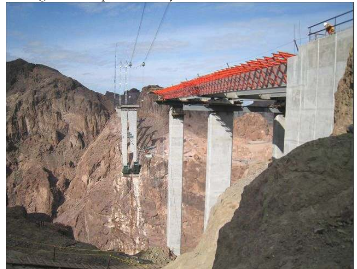
A January, '08 view of two, 400' tall piers bearing on the arches' thrust-blocks
