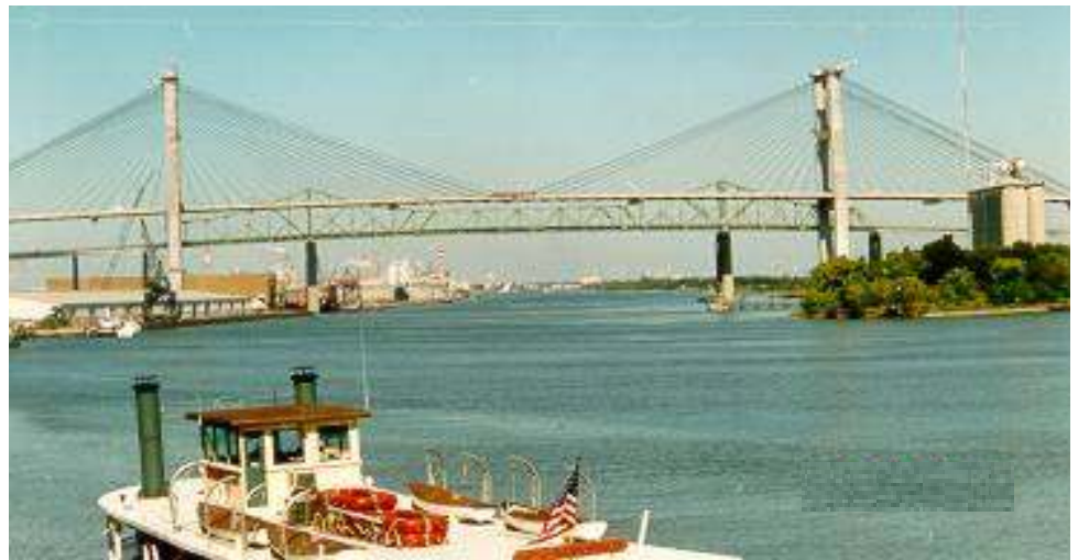
Figure 1: The view, down river, of the new cable-stayed bridge, under construction, framing the replaced steel truss, beyond.
