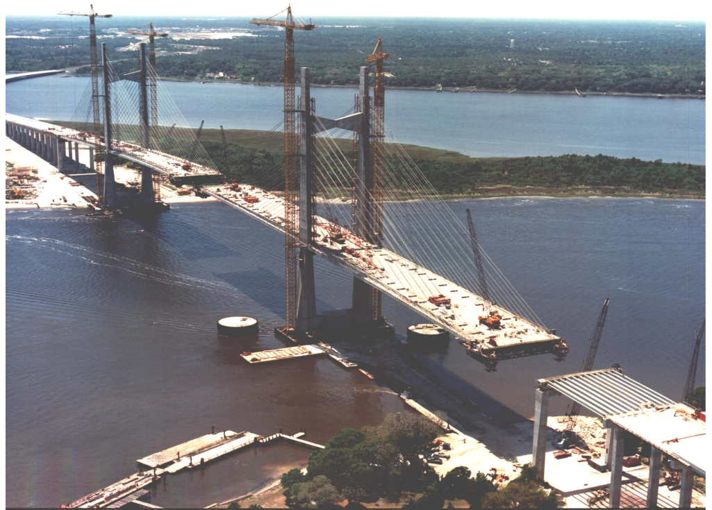
FIGURE 4: BOTTOM BOW-TIES OMITTED DURING CONSTRUCTION PERMITTING CRAWLER CRANES MOVEMENT ON DECK.
