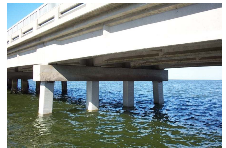
FIGURE 6: Painted, UV protected piles
