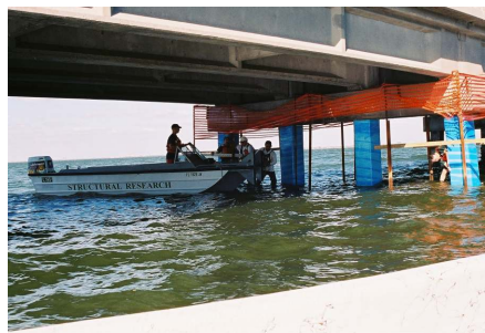
FIGURE 5: Piles wrapped above and below water
