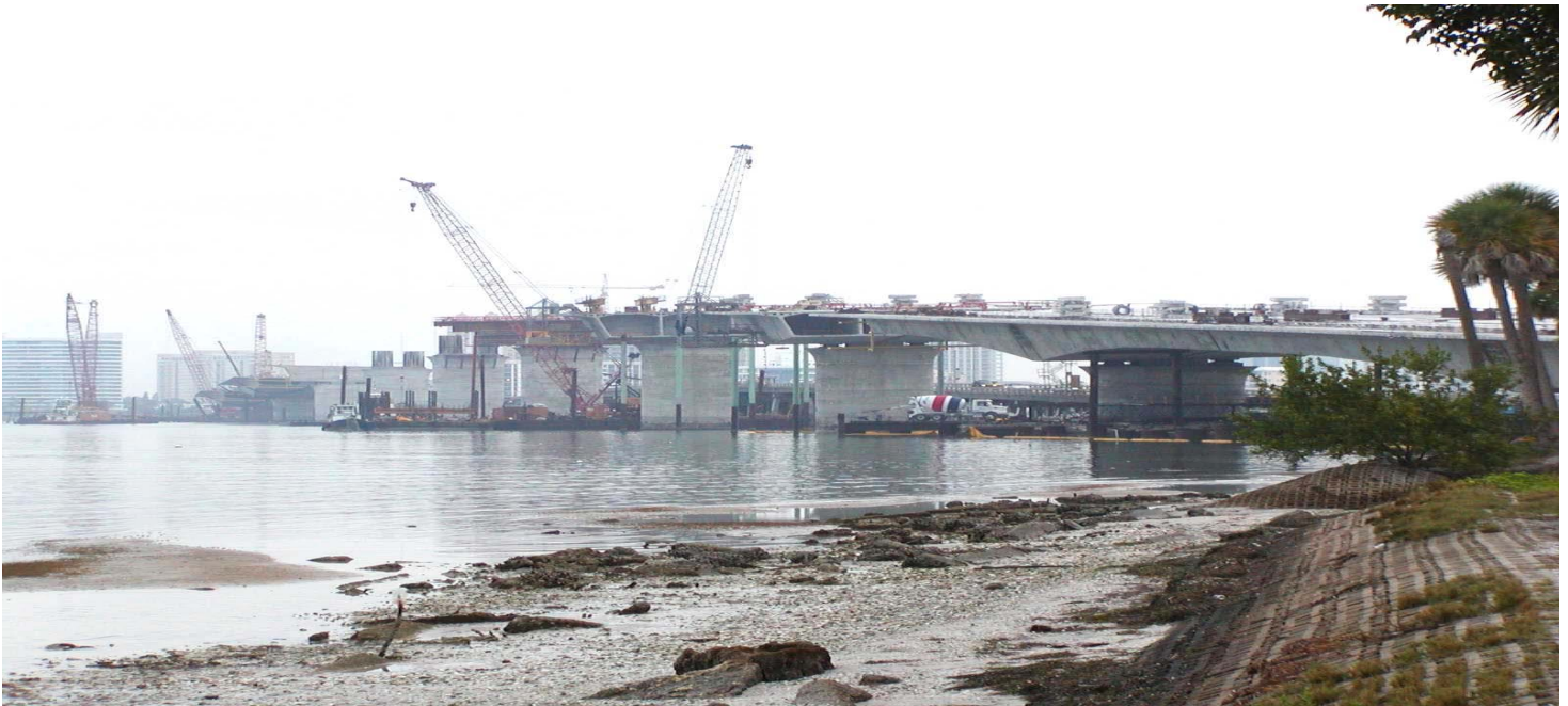
Mainland view of the new Ringling Bridge under construction in Sarasota, FL 11/21/02
